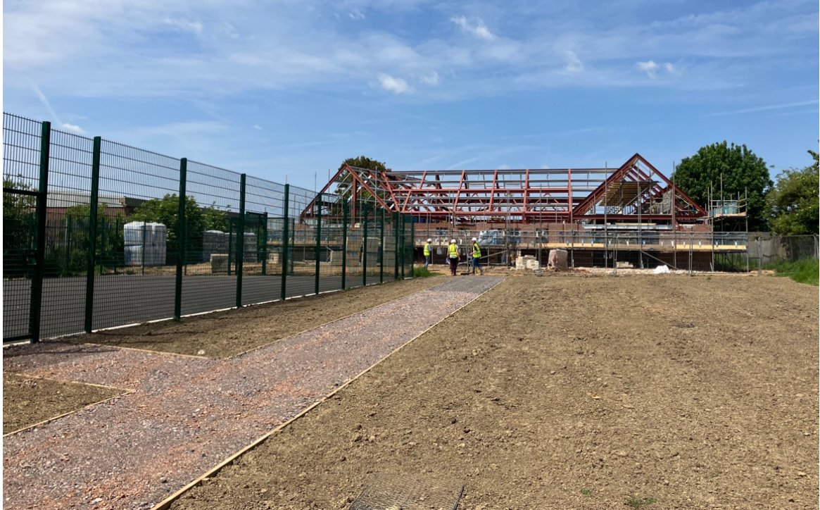
Photo of the new Keystone Centre and MUGA in Eldon Way Littlehampton under construction
